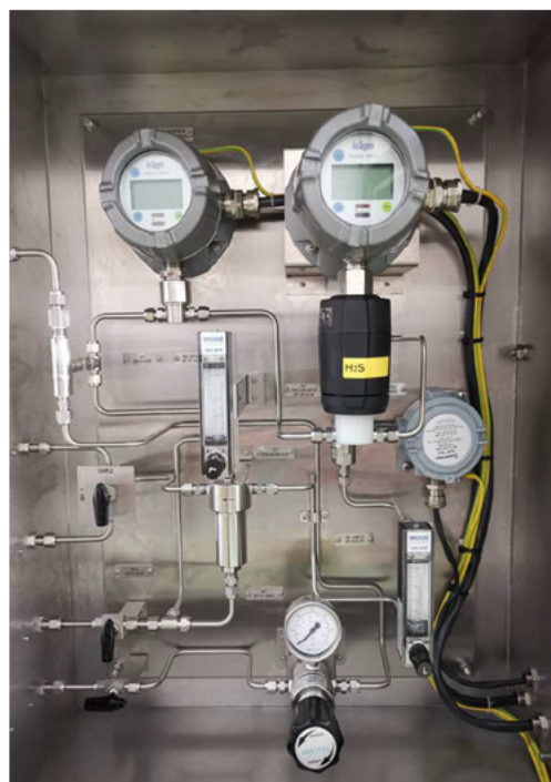
Figure 8 – Typical Aspiration System
